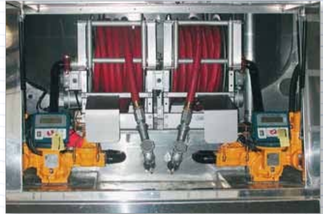
Nozzle Holders that drain directly into below floor collection tank
